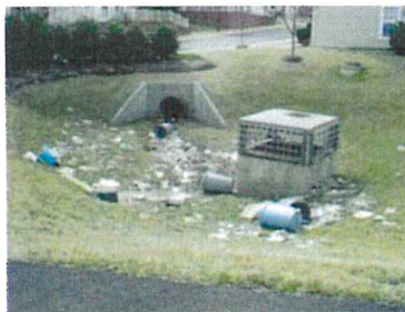
Basin inlet in background and outlet structure with trash rack in center, which has been helpful in preventing debris from being discharged.
