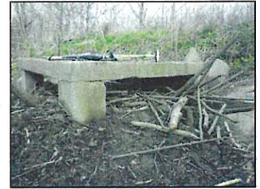
Outlet structure blocked with sediment and debris
