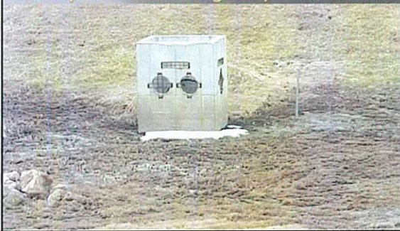
The Outlet Structure With Trash Screens. The Top Of The Outlet Is Open For Emergency Overflow
