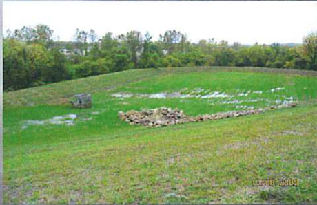
Walmart Basin With A Forebay To Slow Flow And Catch Sediment
