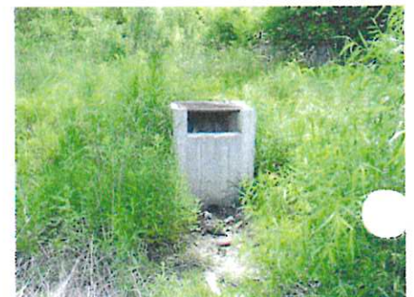
Detention basin outlet structure; mowing here would be helpful
