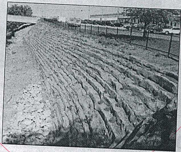
JIM BASKAS Shown is the construction work that has been done on Three Mile Creek.
