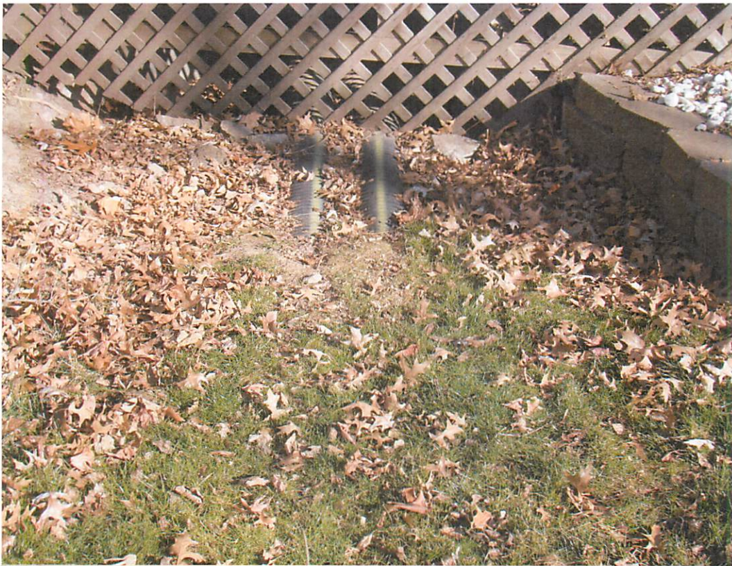
#5: Photos shows two additional drainage tubes that divert water into the storm drain at 1106 South 14th St.
