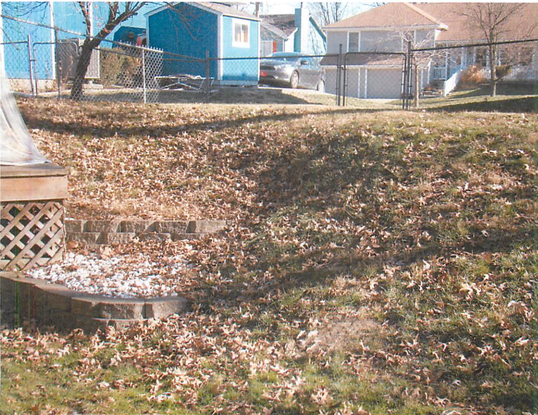
#6: Shows the step drop off in elevation from the northside gate entry looking directly east. Water also runs into this storm drain from above as shown by the ruts in the yard.
