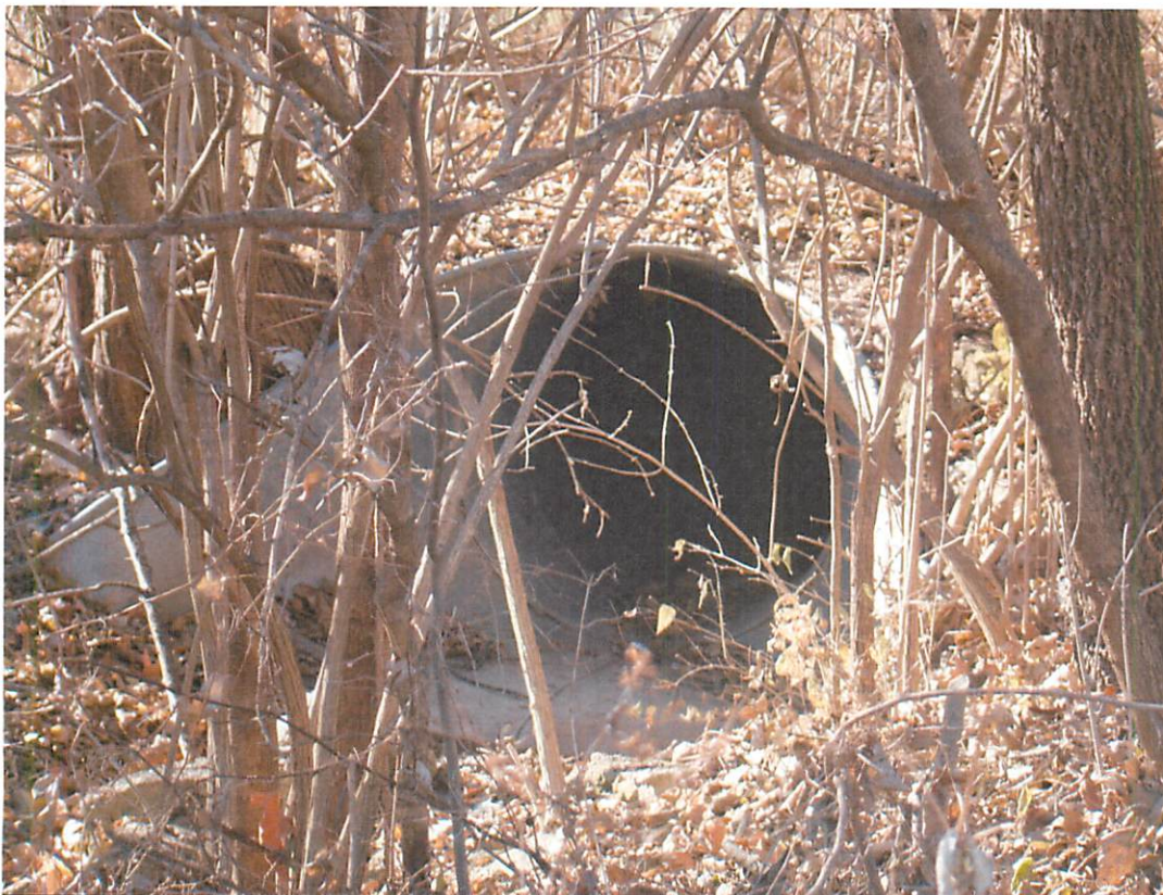
#8: The water then exits through this storm drain located between 1110 & 1028 Madison St.
