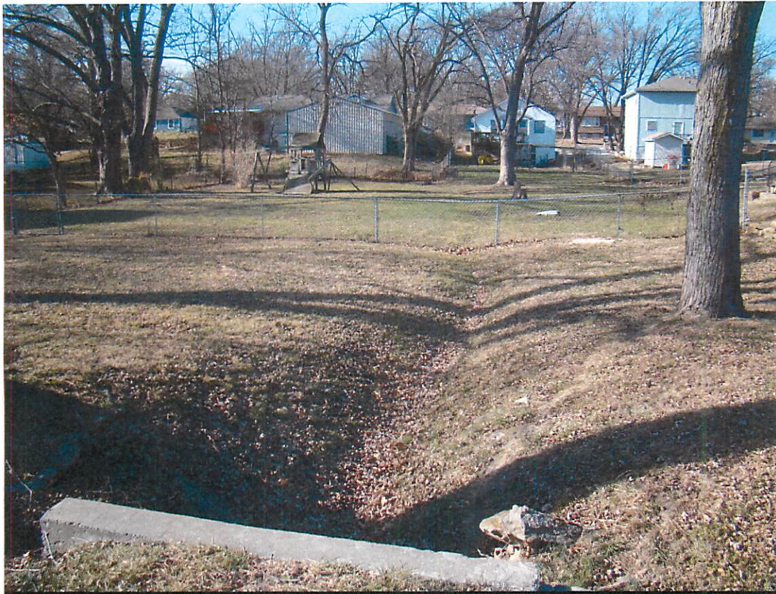
#11: Water from Madison St continues to flow eastward into this area adjacent to 910 Washington St. During periods of continuous rainfall this area floods
