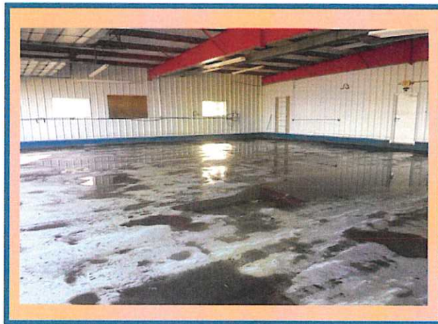
Hangar after Water Receded - March 2019
