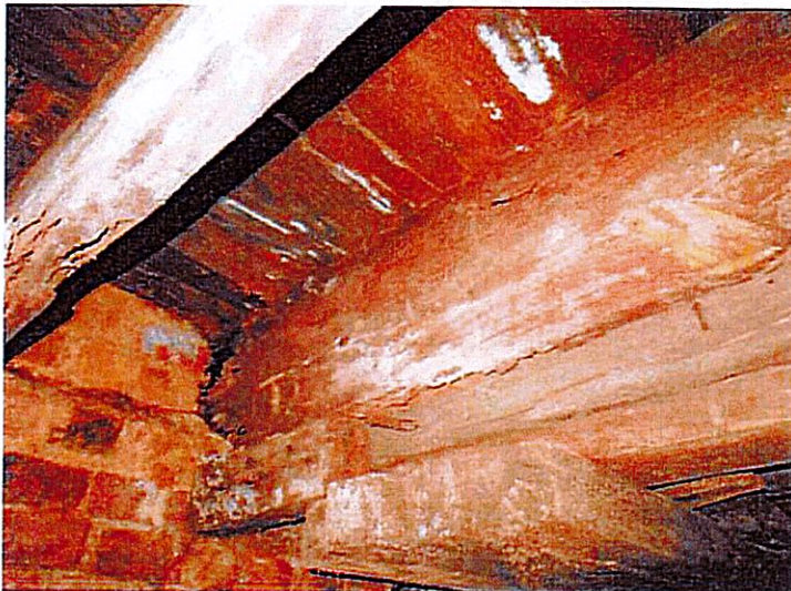
14. Extensive deterioration, rot, and termite damage in the joists closer to the south end of the east side.
