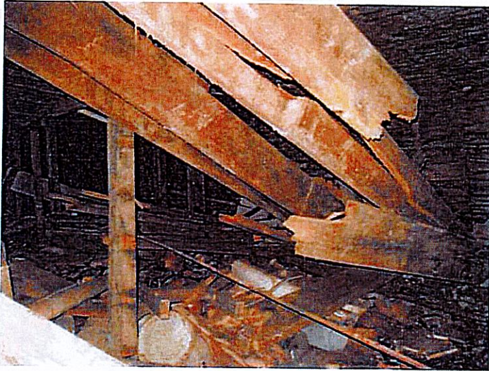
7. Collapsed wood framing as seen in the basement.
