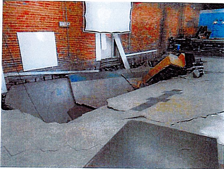
5. Collapsed floor in the western half of the building as seen from the southeast.
