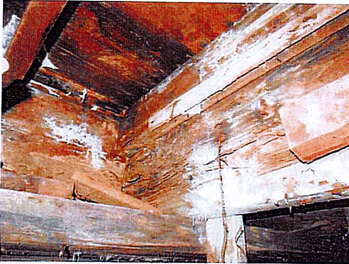
11. Extensive deterioration, rot, and termite damage in the floor joist framing along the east wall.
