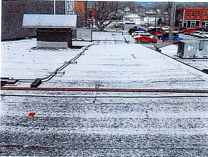
27. Low angle view of the roof showing the sag present in the roofing.
