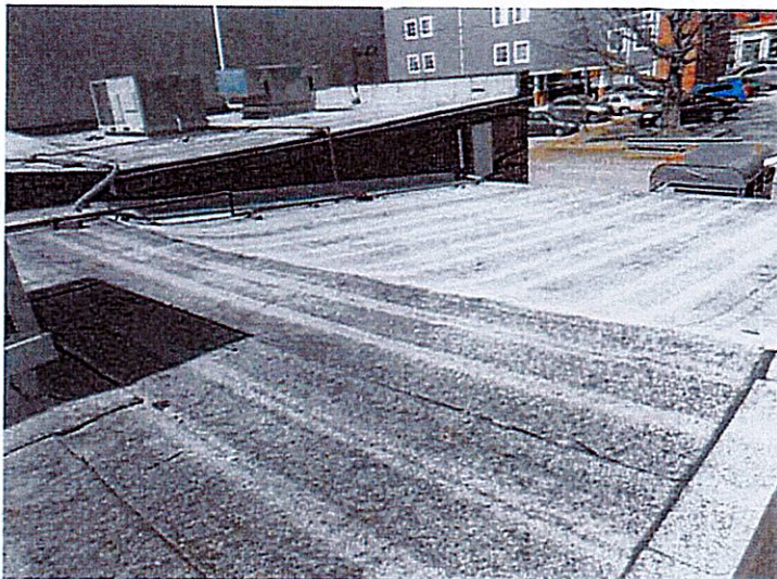
24. Northern portion of the east roof with the western half of the building in the background.
