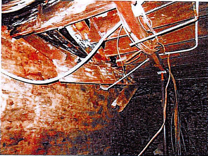
15. Partially collapsed floor framing at the old stairway location located at the southeast corner.
