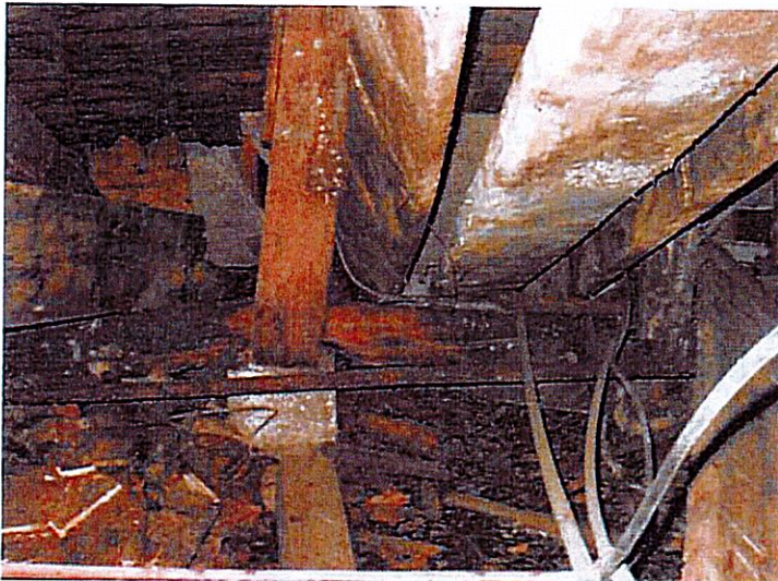
8. Close-up of deterioration and rot in the center support beam.
