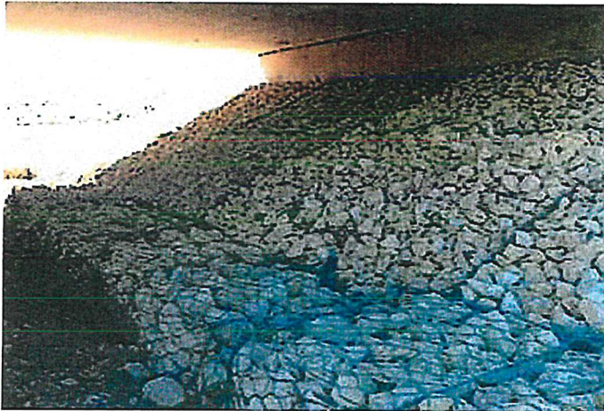
The City places riprap under bridges to protect the structure from erosion
