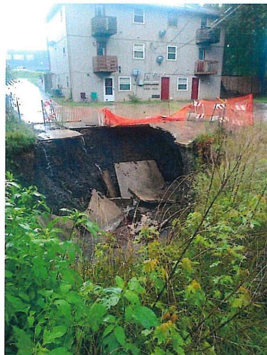
Sinkhole Near Apartments
