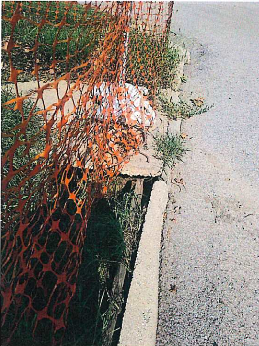
Sinkhole Undercutting the Street
