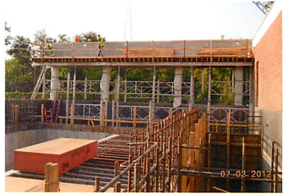
Construction crews continue work on the $4.3 million wastewater disinfection project at the City's water treatment plant. Work is scheduled to be done by the end of the year.
