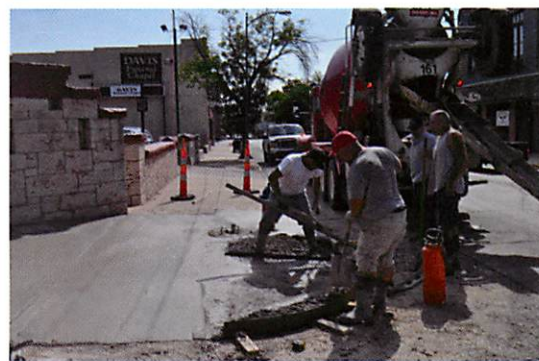
Workers construct new curb ramps in anticipation of new traffic signals at the intersection of Sixth and Shawnee streets
